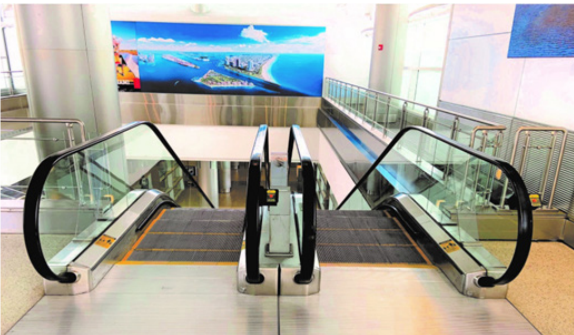
Escalators at MIA
